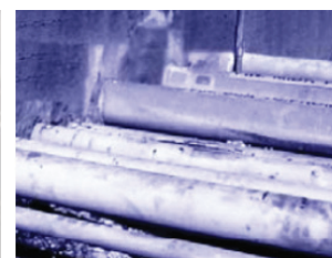
Piping through the wall
